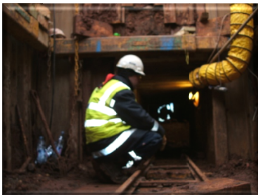
Tunnel for 750mm MP gas main Leicester 2010 working for Duffy tunnelling and National Grid Gas
